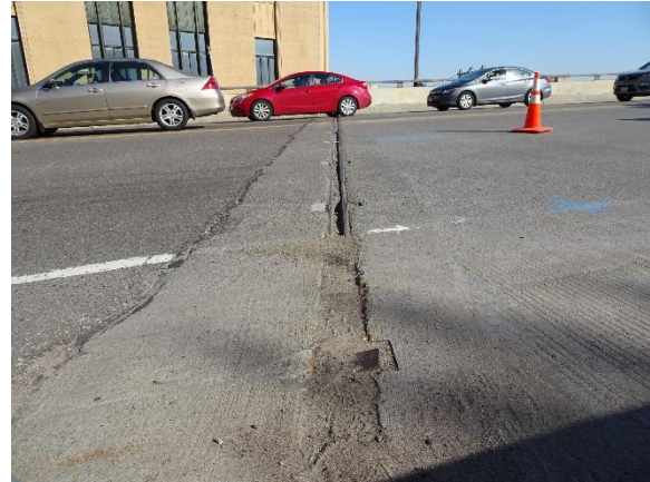
Figure 4.80. South approach strip seal joint with missing plow fingers.
