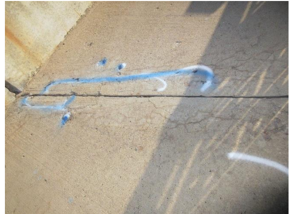
Figure 4.24. Distress similar to D-cracking at poured sealant joints.
