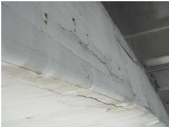
Figure 4.48. Arch rib corner delamination
