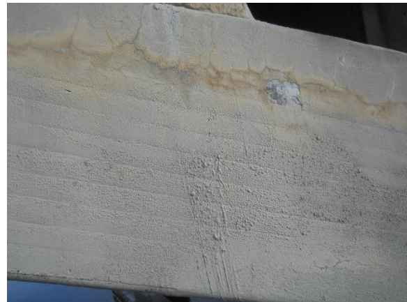
Figure 4.49. Arch rib deteriorated concrete repair.
