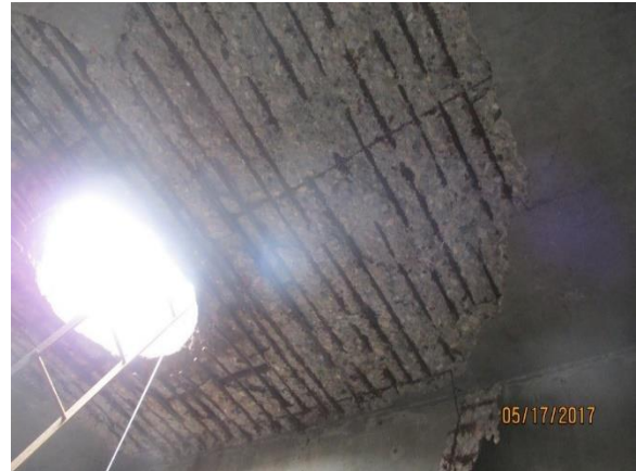
Figure 4.17. Slab underside spalls and rebar section loss at manholes in southbound lane.
