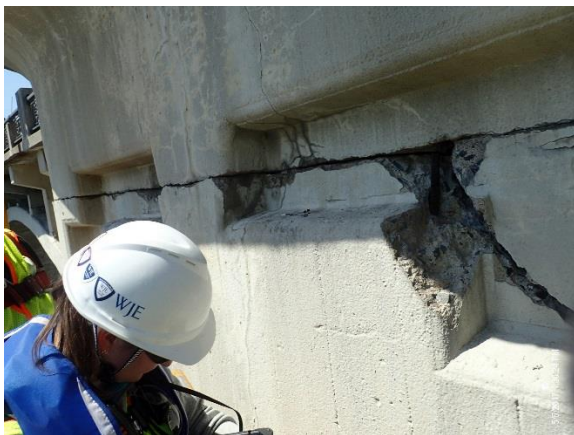
Figure 5.20. Pier 8, downstream face, sliding along horizontal joint near top.
