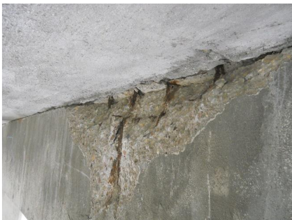
Figure 4.35. Deep cap beam spall with exposed vertical dowels into deck.
