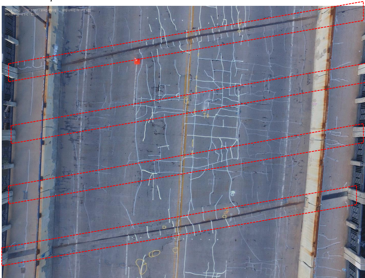
Figure 4.18. Sample aerial drone image of deck span 4A to 4D. Deck cracks were field-marked with non-permanent white spray chalk. Delaminations were circled in yellow. Locations of cap beams below indicated by dotted red lines.
