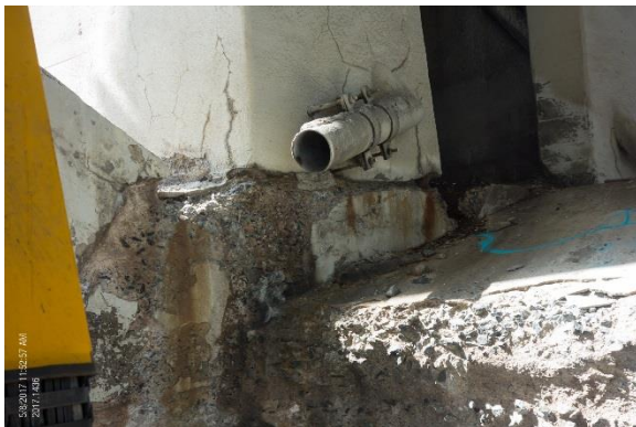
Figure 4.71. Drain outfall at Pier 2 and concrete deterioration below.
