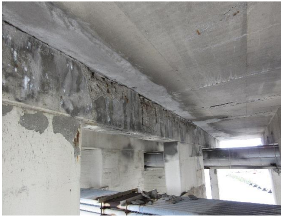
Figure 5.31. Spalling along top corner of cap beam.
