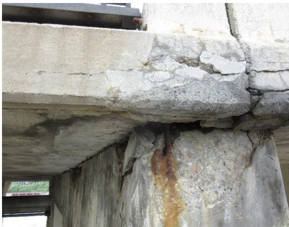
Figure 5.42. Spalling of deck fascia at deck joint.
