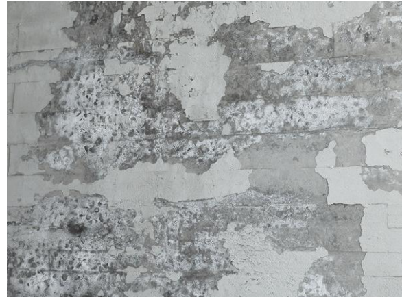
Figure 4.7. Freeze-Thaw Condition State 2. Surface scaling without substantial material loss.
