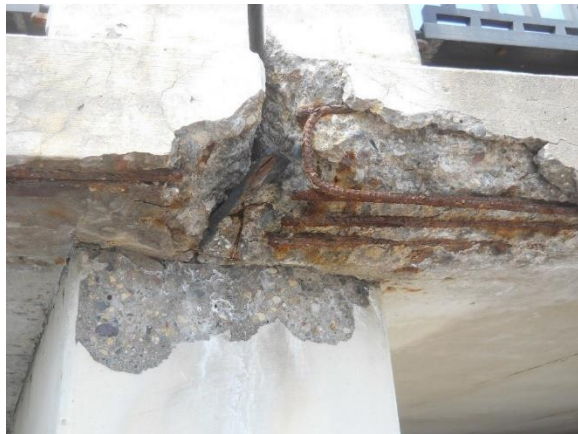
Figure 4.12. Downstream deck edge spall at expansion joint.
