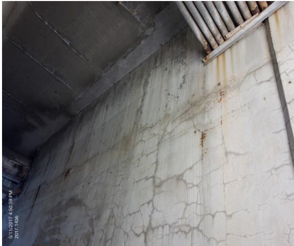
Figure 4.44. Map-cracked repair material.
