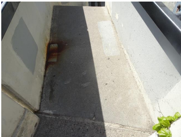
Figure 4.113. North vertical circulation staircase rust stains and cracks at walkway to bridge.
