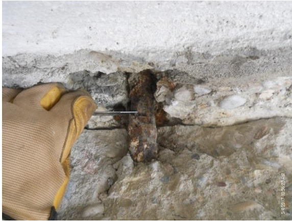
Figure 5.35. Close-up of vertical dowel, showing corrosion of dowel and direct contact between repair concrete and top of cap beam.
