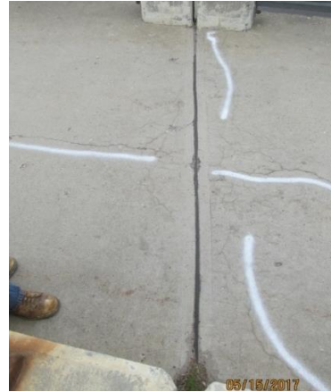
Figure 4.22. Longitudinal crack along upstream sidewalk.
