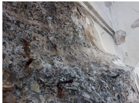
Figure 4.9. Freeze-Thaw Condition State 4. Concrete disintegration and erosion extending greater than 2 inches in depth from original section, or exposed bars.
