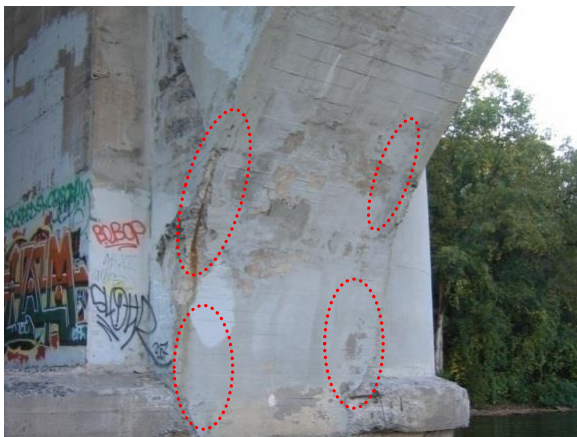
a) Franklin Avenue Bridge (2008) - View of freeze thaw deterioration near base of arch ribs (circled).
