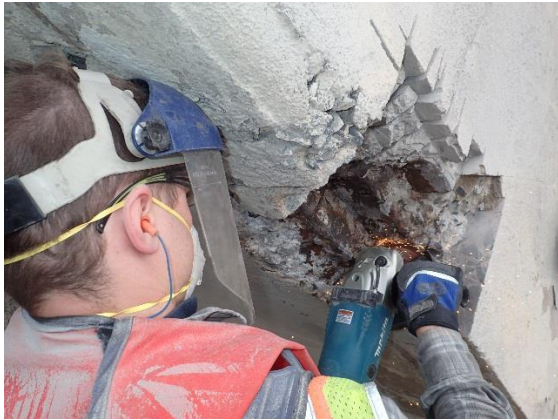
Figure 3.3. Sample removed from delaminated and spalling arch rib corner by cutting edge of angle.
