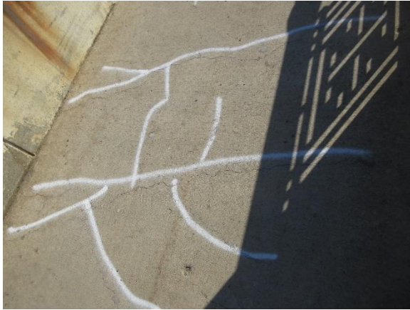
Figure 4.21. Sidewalk cracks over cap beam.
