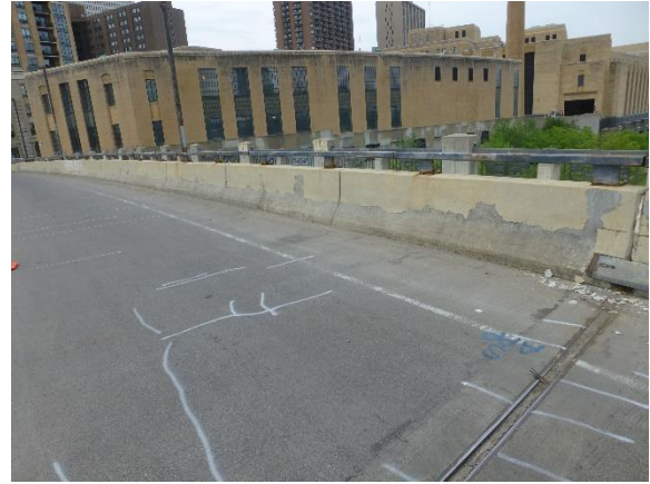
Figure 4.108. Traffic barrier failed coating.
