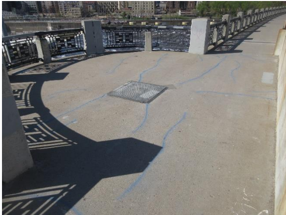
Figure 4.23. Cracks originating from catwalk access hatch.
