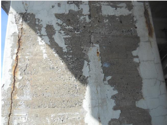
Figure 4.40. Spandrel column vertical cracking, coating failure and eroded concrete surface.
