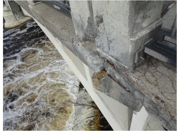
Figure 4.100. Deep spall in deck fascia below railing post.
