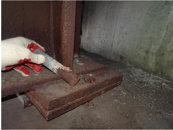
Figure 4.81. South abutment fixed bearing fractured anchor bolt.
