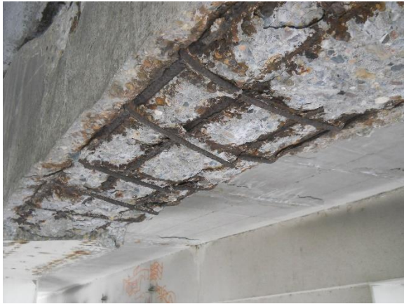
Figure 4.33. Cap beam stirrups corroded through.
