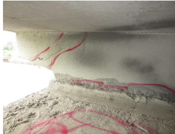
Figure 5.41. Shear or torsional cracking in cap beam in Span 7, downstream side.
