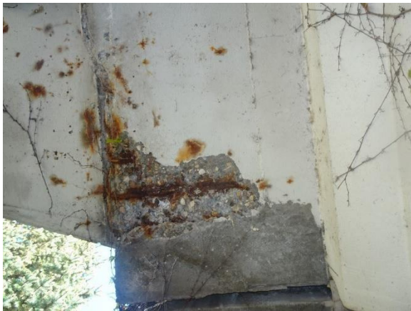
Figure 4.89. North approach slab underside spall near the north abutment.
