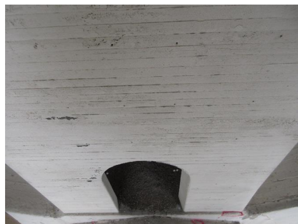
Figure 4.64. Typical appearance of pier wall in good condition. Note original form board texture.
