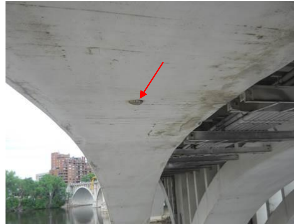
Figure 2.16. Example of hole (arrow) through arch rib for previous drain pipe penetration.
