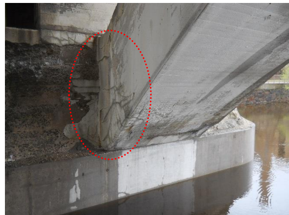
b) 3rd Avenue Bridge (2017) - View of freeze thaw deterioration near base of arch rib.
