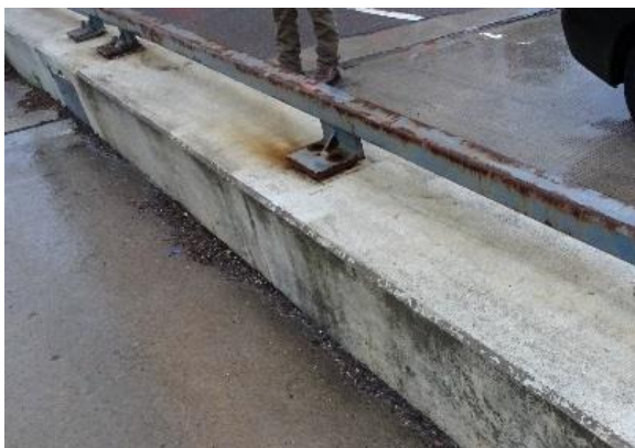
Figure 4.111. Traffic barrier metal railing missing fasteners.
