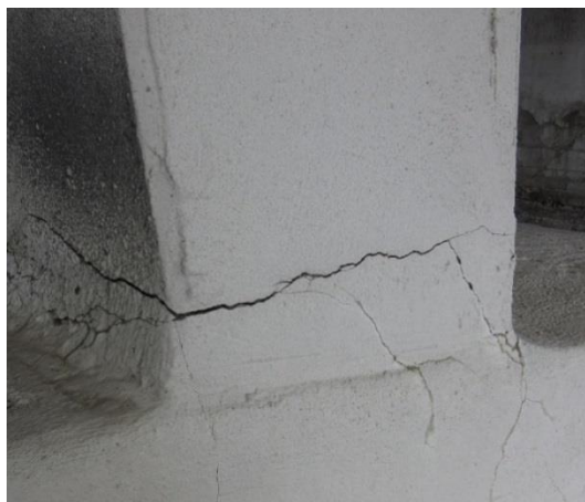
Figure 5.26. Spandrel column structural distress, distress category 1.
