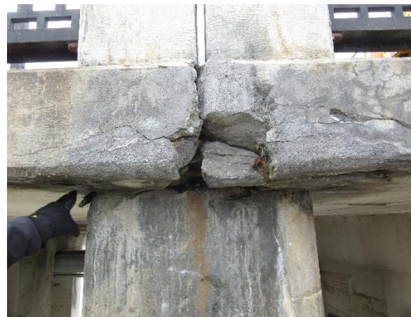
Figure 5.43. Spalling of deck fascia at deck joint.
