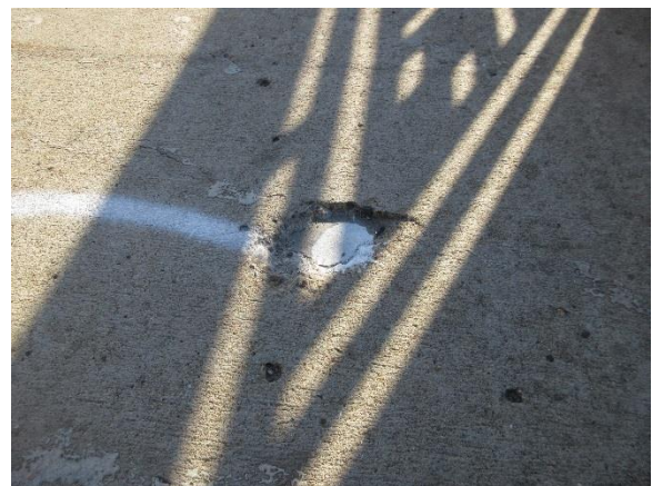
Figure 4.26. Small aggregate pop-out.
