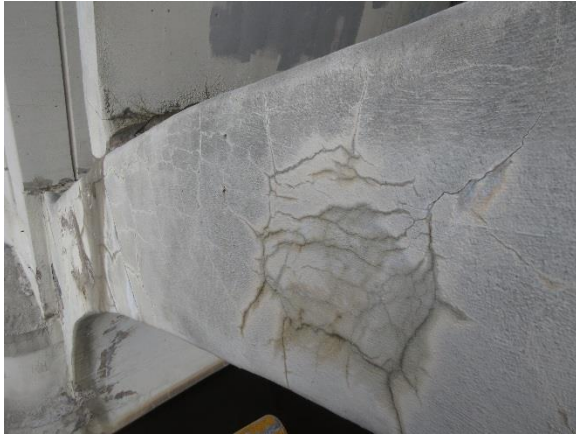
Figure 4.6. Freeze-Thaw Condition State 1. Map cracking and moisture staining only.
