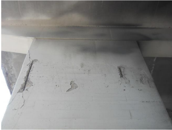
Figure 4.38. Spandrel column spalls at vertical rebar.
