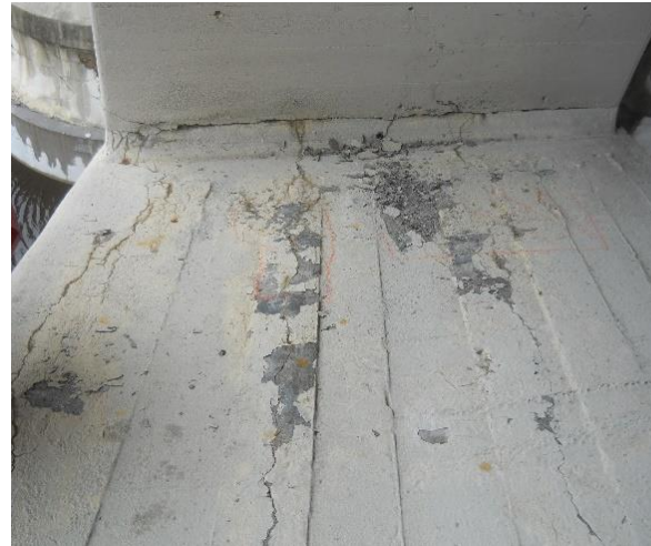
Figure 4.53. Arch rib topside cracks aligned with Melan truss angles.
