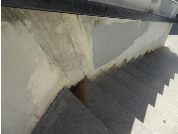
Figure 4.115. North vertical circulation staircase rust stains at stair treads.
