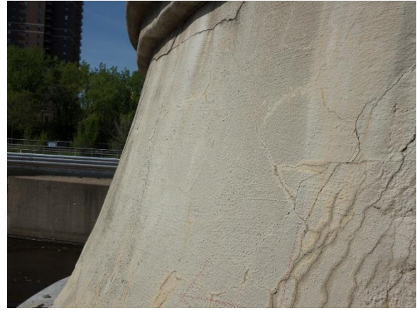
Figure 4.3. Coating Condition State 2. Fair, some distress, including cracking and evidence of moisture movement behind coating.
