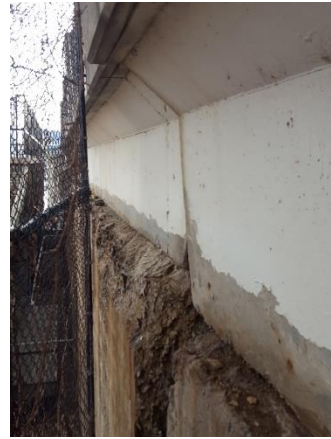
Figure 4.95. North approach, downstream side, cap on top of original retaining wall rotated outward (left in photo).
