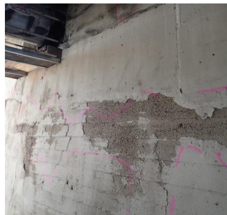
Figure 4.43. Delaminations along vertical and horizontal bars in original concrete.
