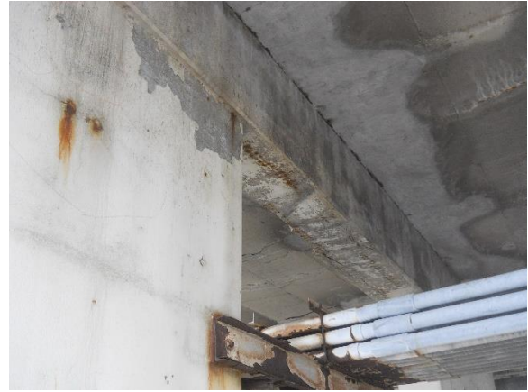
Figure 4.32. Cap beam underside delamination.
