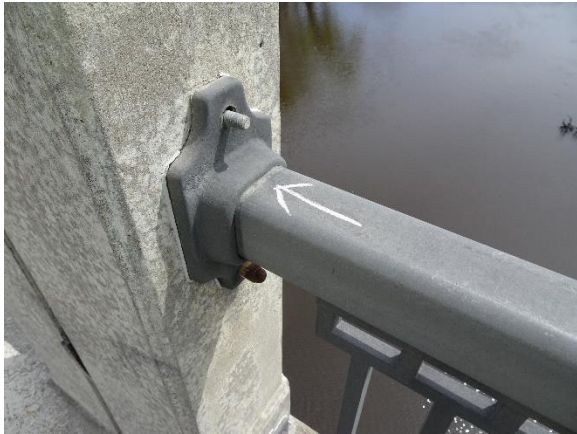
Figure 4.101. Aluminum railing connection missing fastener.
