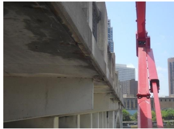
Figure 4.11. Upstream deck edge condition.
