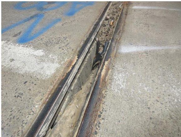
Figure 4.91. North approach strip seal gland tear.
