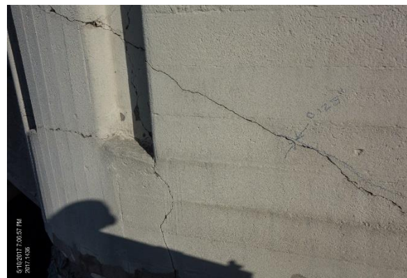
Figure 5.25. Pier 1, upstream face, close-up of shear cracking.
