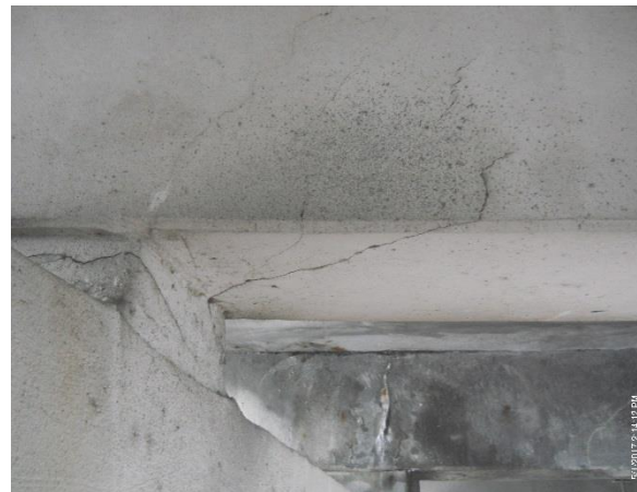
Figure 5.39. Shear or torsional cracking in cap beam in Span 1, downstream side.
