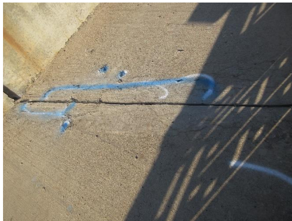
Figure 4.27. Concrete repair and delamination at poured seal.
