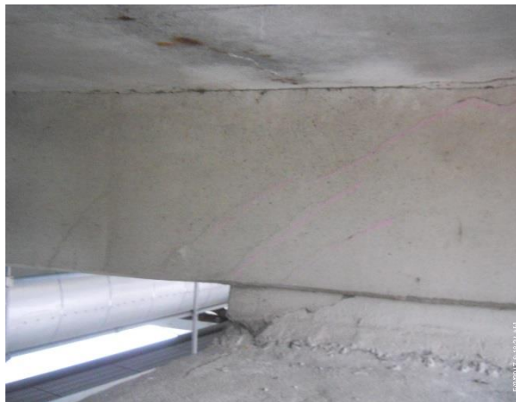
Figure 5.38. Shear or torsional cracking in cap beam in Span 1, downstream side.
