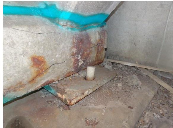
Figure 4.93. Precast beam concrete distress at north abutment.
