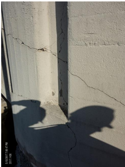
Figure 4.67. Wide diagonal crack at Pier 1, upstream face.
