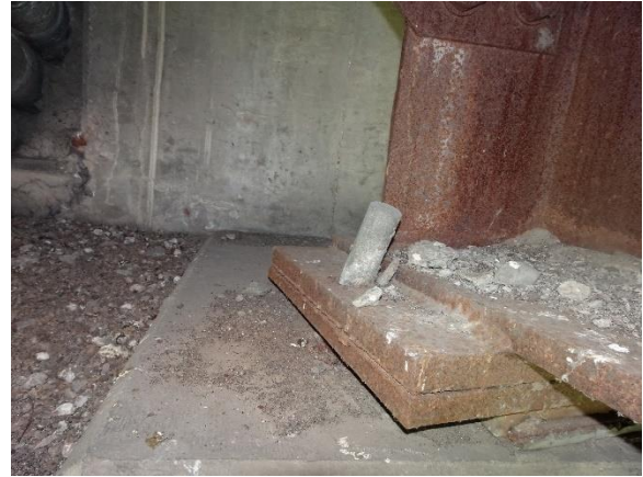
Figure 4.82. South abutment fixed bearing bent or rotated anchor bolt.
