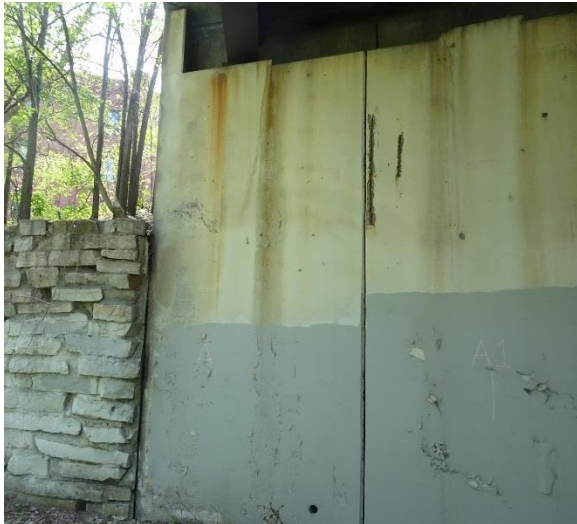
Figure 4.87. South abutment spalls.
