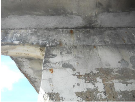
Figure 4.31. Cap beam conditions under expansion joints.
