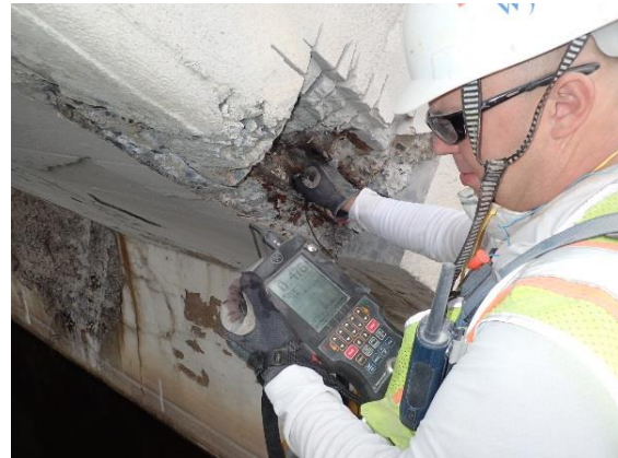
Figure 3.17. Ultrasonic thickness measurement on Melan truss angle in delaminated and spalling corner of arch rib.
