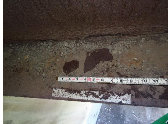
Figure 4.86. South approach, tape adhesion test of weathering steel patina in poor condition and flaking (CS4 rating).
