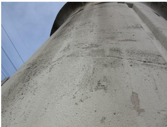
Figure 4.4. Coating Condition State 3. Flaking and small areas of debonding.
