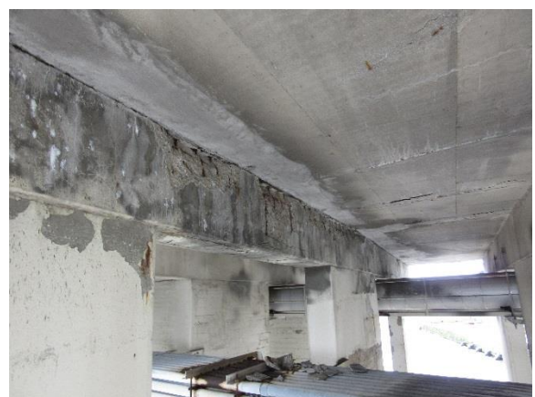
Figure 4.36. Deep spalling along top corner of cap beam.
