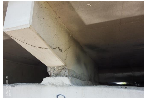
Figure 5.29. Spandrel wall structural distress, distress category 3.
