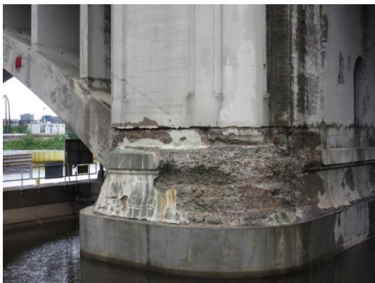
Figure 5.24. Pier 1, upstream face, shear cracking.
