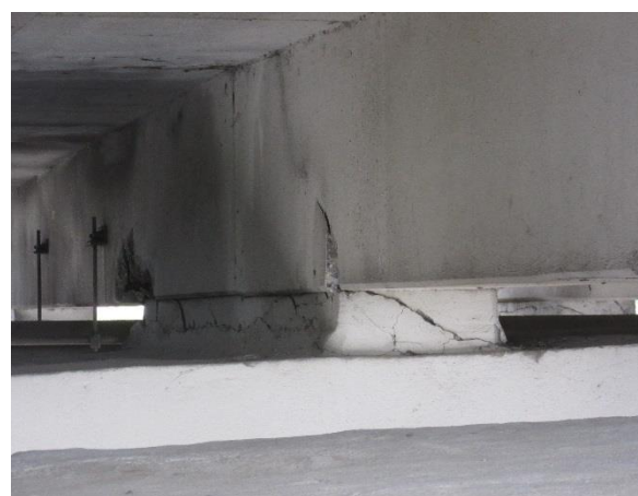
Figure 5.27. Spandrel column structural distress, distress category 2.
