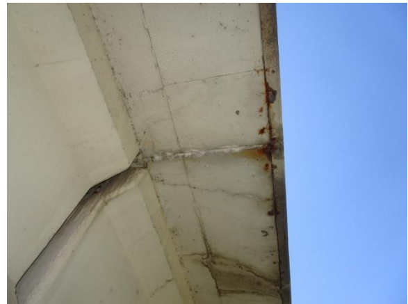
Figure 4.90. North approach slab underside diagonal cracking and efflorescence at the north bent.
