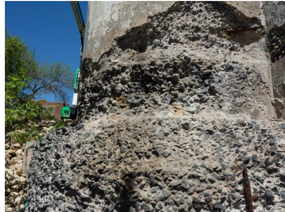
Figure 4.70. Freeze thaw distress at the base of Pier 8.
