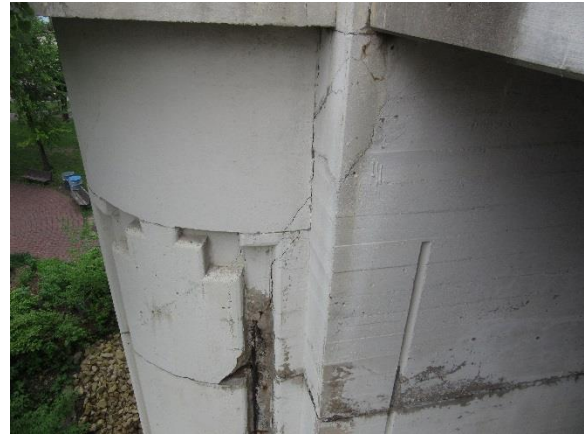
Figure 5.23. Pier 8, upstream face, close-up of shear cracking extending from deck.
