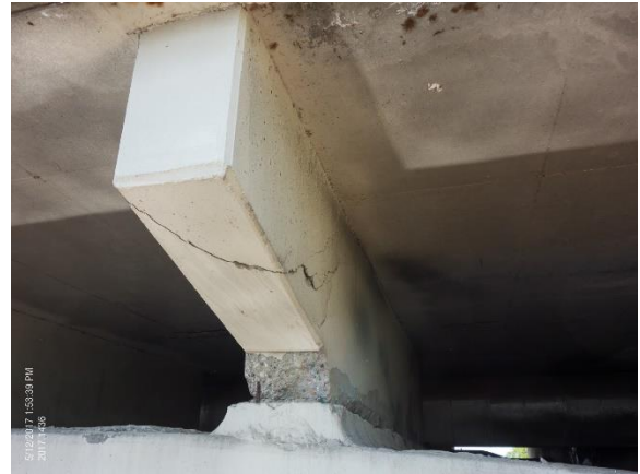
Figure 4.34. Cap beam shear or torsional crack.
