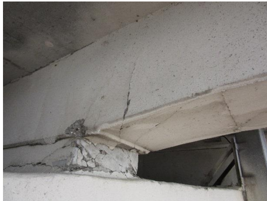
Figure 5.28. Spandrel column structural distress, distress category 3.
