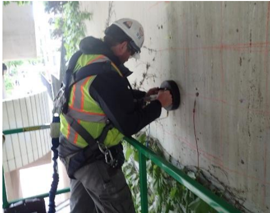
Figure 3.10. Corrosion rate survey (north abutment).
