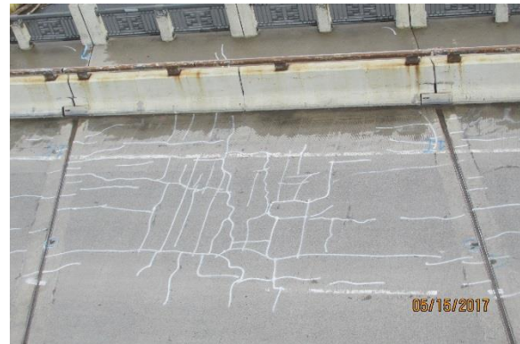
Figure 5.11. Photograph within arch span showing seals in roadway and poured sealant joints in sidewalk.
