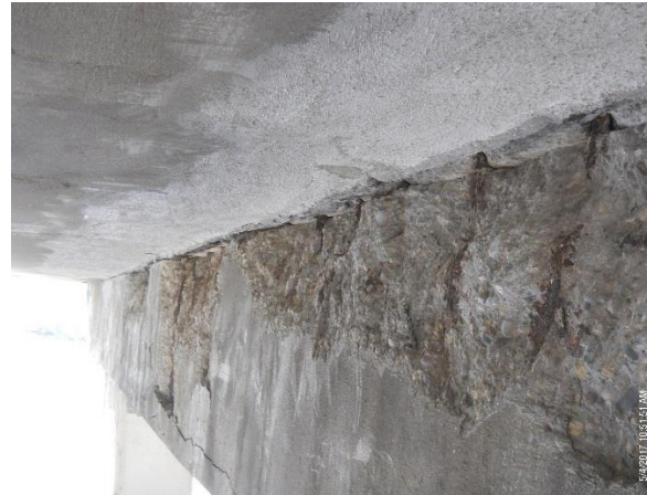
Figure 5.32. Close-up of cap beam spalling, showing exposed vertical dowels.
