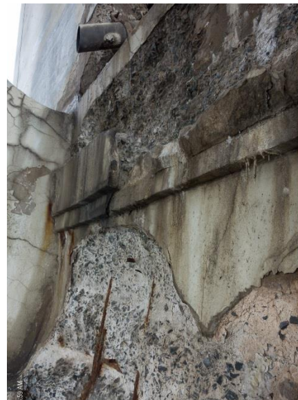
Figure 4.72. Drain outfall at Pier 6 and concrete deterioration below.
