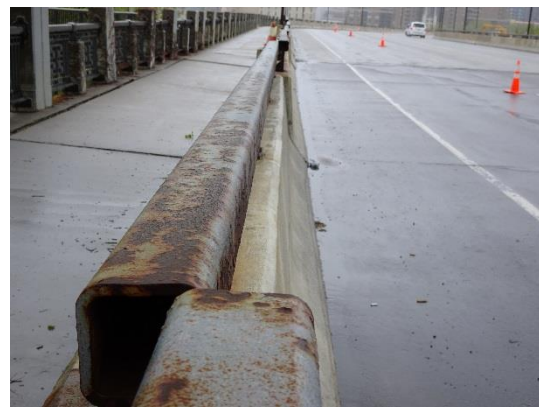
Figure 4.112. Traffic barrier metal railing out of alignment.
