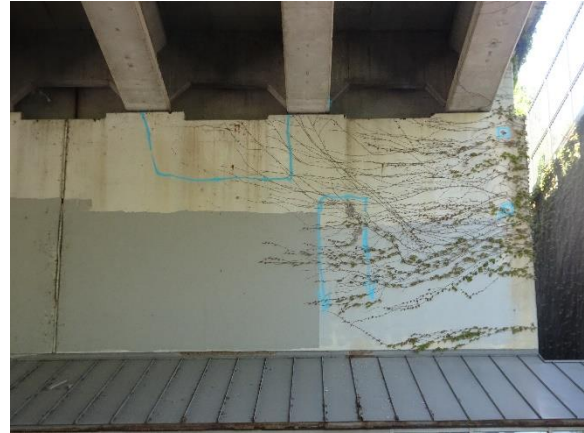
Figure 4.98. North abutment delaminations.
