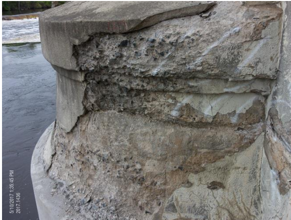
Figure 4.69. Freeze thaw distress at the base of Pier 2.
