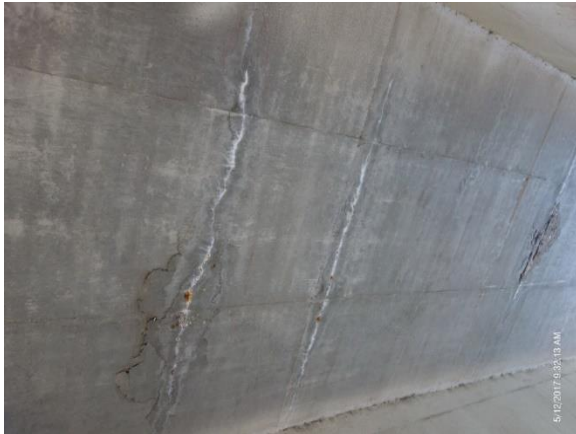
Figure 4.16. Slab underside cracks and delaminations throughout deck.
