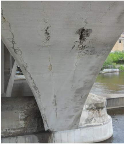
Figure 4.54. Arch rib underside cracks aligned with Melan truss angles.
