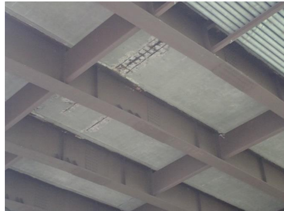
Figure 4.78. South approach slab underside spalls near south bent.
