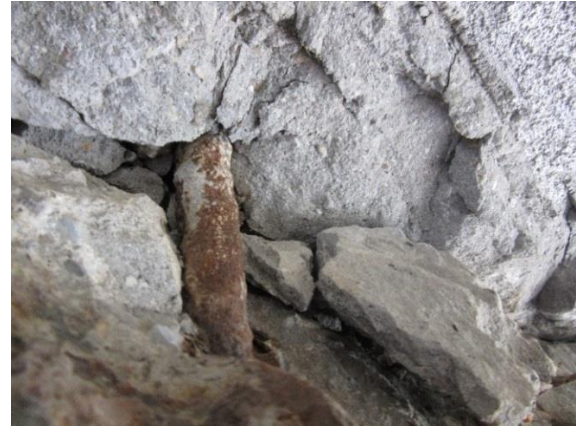
Figure 5.36. Close-up of vertical dowel, showing repair concrete tight against dowel.
