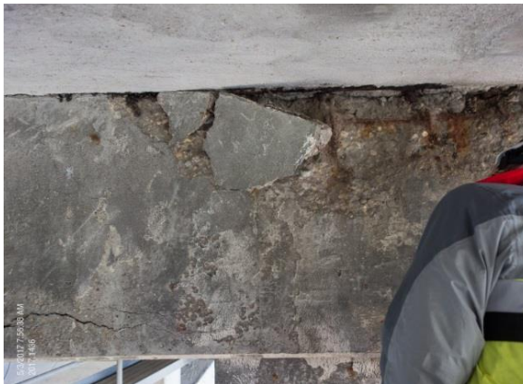
Figure 5.33. Cap beam spall that was developing at the time of the inspection.
