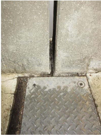
Figure 5.12. Termination of strip seal at inside face of railing post, with original poured sealant joint visible between posts.
