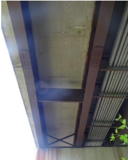
Figure 4.77. South approach transverse cracks on slab underside along sidewalk.
