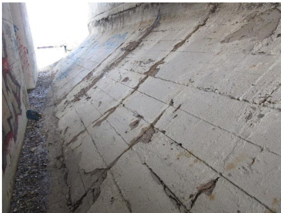
Figure 4.58. Barrel arch topside cracks aligned with Melan truss angles.
