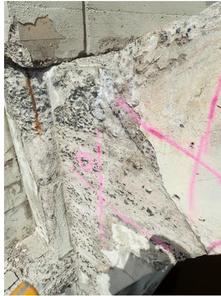
Figure 4.61. Barrel arch freeze-thaw deterioration at arch spring line.
