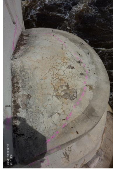
Figure 4.74. Deteriorated repair material at the base of Pier 3.
