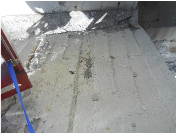
Figure 4.56. Arch rib transverse crack on topside.
