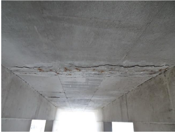
Figure 4.14. Slab underside delamination at centerline of deck.
