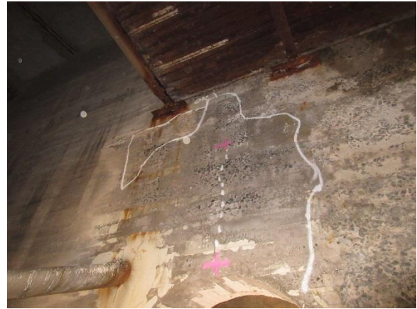
Figure 4.66. Deteriorated concrete below access platform on the inside of Pier 1.
