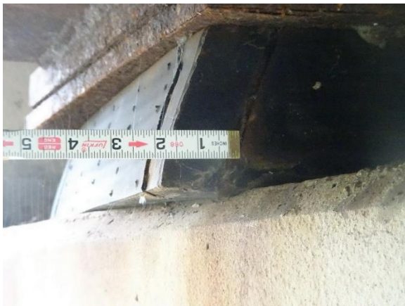
Figure 4.83. Pier 1 expansion bearing pad deformed and displaced off edge of concrete support.
