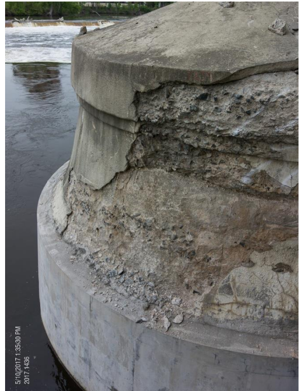
b) 3rd Avenue Bridge (2017) - Freeze thaw distress extending many feet above water level, and a concrete repair jacket was previously installed at this pier.
