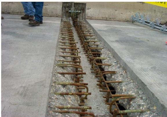
Figure 5.13. Construction photograph from 2003 joint replacement project (provided by MnDOT). Note vertical dowels exposed in repair area.
