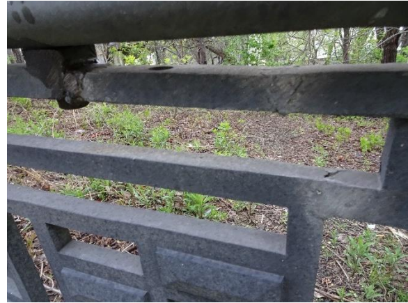
Figure 4.106. Pedestrian railing unsound metal repairs.
