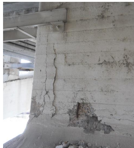
Figure 4.47. Spandrel column corner delamination near utility duct support.
