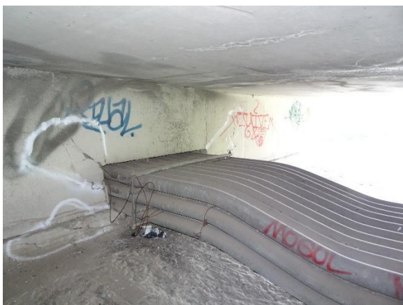
Figure 4.42. Cracks emanating from corners of utility duct opening.
