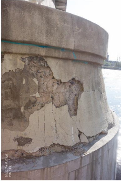
Figure 4.73. Deteriorated repair material at the base of Pier 2.
