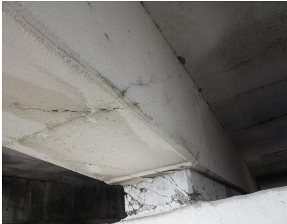
Figure 5.40. Shear or torsional cracking in cap beam in Span 1, upstream side.
