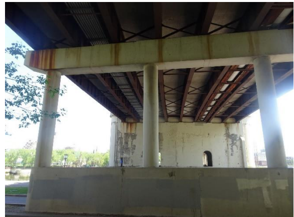
Figure 4.88. South bent pier cap rust stains.
