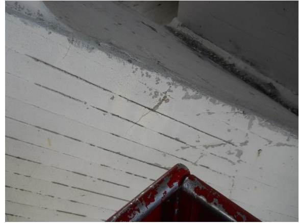
Figure 4.55. Arch rib transverse crack on upstream face.
