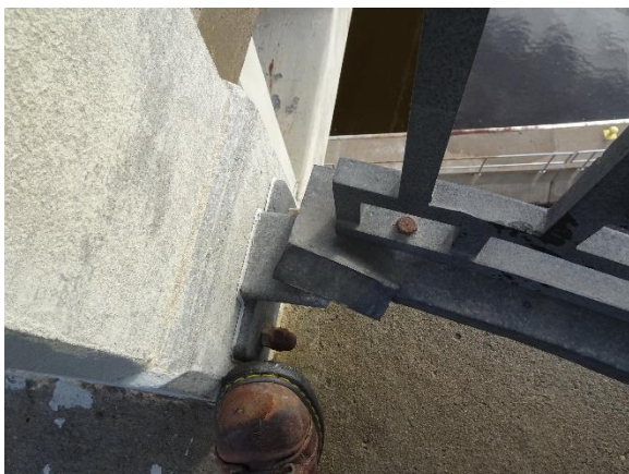
Figure 4.103. Bottom railing distorted, likely from impact.
