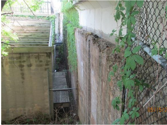
Figure 4.97. View looking south along downstream retaining wall. Note freeze-thaw damage at top of original concrete.
