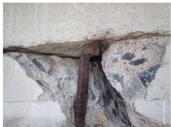
Figure 5.21. Pier 8, downstream face, fractured bar across horizontal joint near top.
