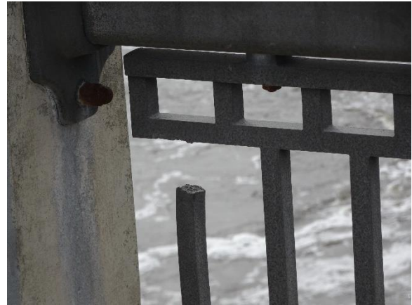
Figure 4.102. Aluminum railing missing member.
