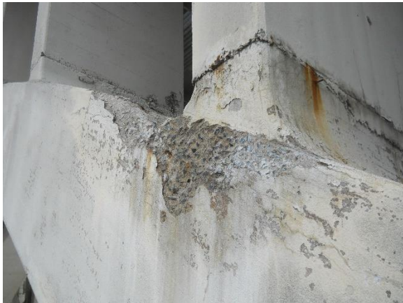
Figure 4.52. Arch rib freeze-thaw deterioration at spandrel column base.
