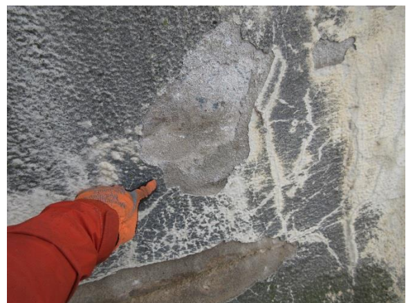
Figure 4.5. Coating Condition State 4. Debonding of large areas of coating.
