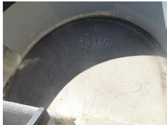
Figure 4.114. North vertical circulation staircase cracks at landing.
