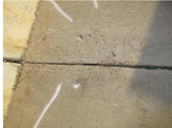
Figure 4.30. Missing section of poured sealant.
