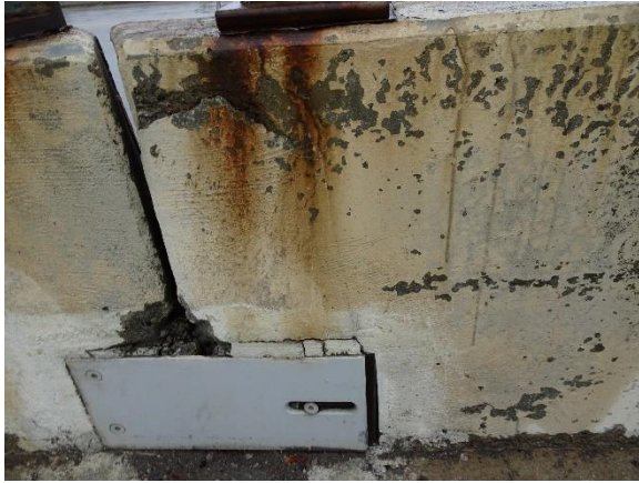
Figure 4.107. Spall in traffic barrier J-rail at expansion joint.
