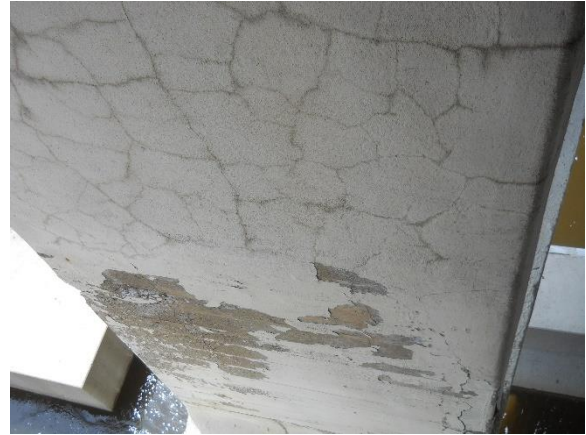
Figure 4.39. Spandrel column map cracking in repair material.
