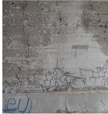
Figure 4.45. Surface erosion of cement paste.
