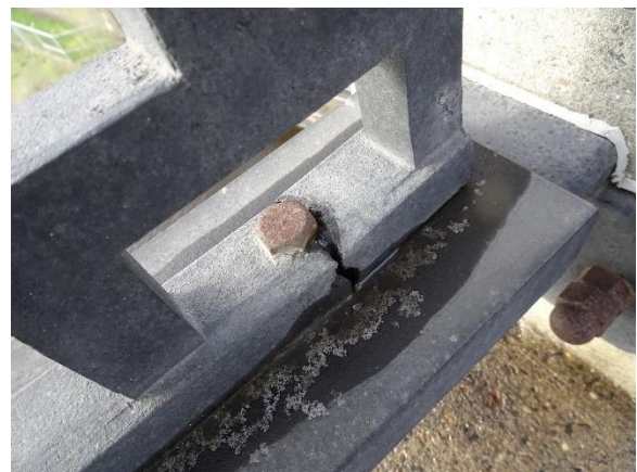
Figure 4.104. Aluminum railing crack.
