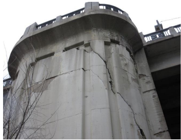
Figure 5.19. Pier 8, close-up of top of downstream face showing wide diagonal cracking.
