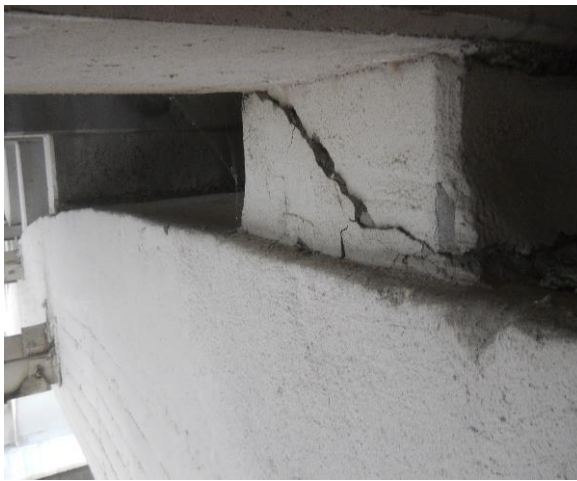
Figure 4.46. Spandrel column shear crack.
