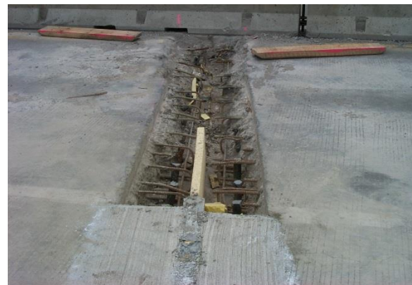
Figure 5.14. Construction photograph from 2003 joint replacement project (provided by MnDOT). Note foam surrounds installed over vertical dowels.
