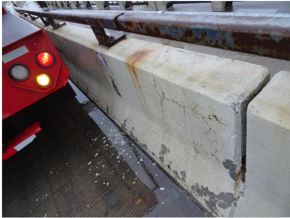
Figure 4.109. Traffic barrier metal railing surface corrosion.
