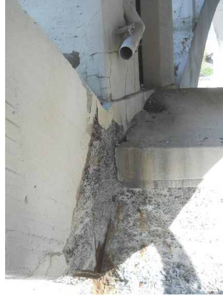
Figure 4.51. Arch rib freeze-thaw deterioration under drain outlet.
