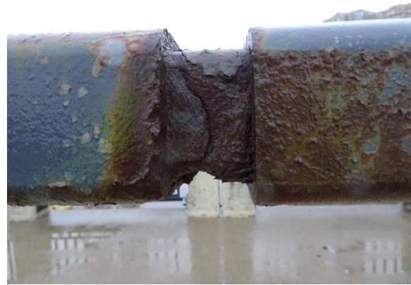
Figure 4.110. Traffic barrier metal railing pack rust at slip joint.
