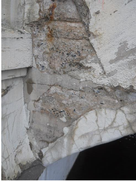
Figure 4.50. Arch rib freeze-thaw deterioration at spring line.
