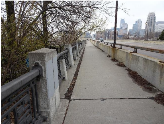
Figure 4.94. North approach, downstream railing leaning outward and gap at sidewalk due to retaining wall cap rotation.
