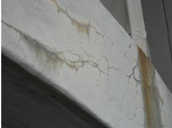
Figure 4.60. Barrel arch deteriorated concrete repair.
