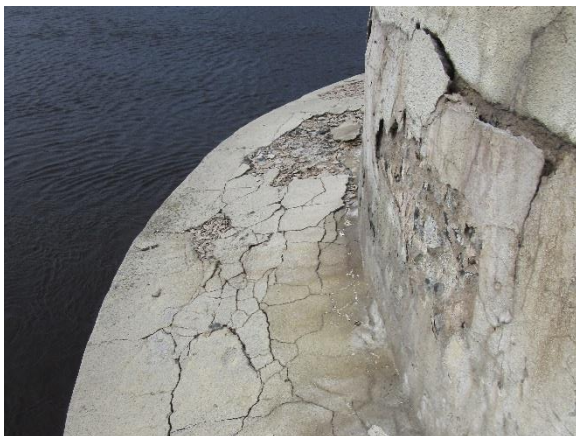
Figure 4.8. Freeze-Thaw Condition State 3. Up to 2 inches (by depth) of concrete deterioration.
