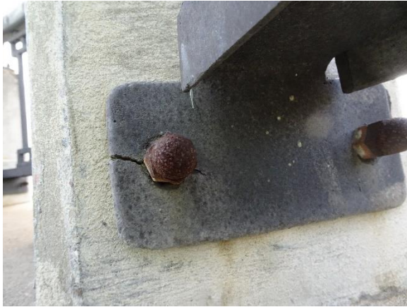
Figure 4.105. Pedestrian railing crack at post connection.
