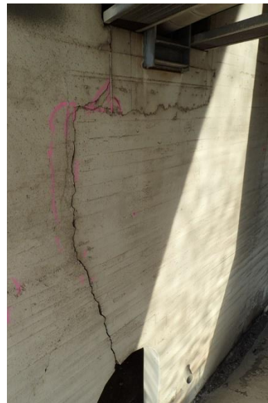
Figure 4.68. Wide crack over arched door opening in Pier 1.
