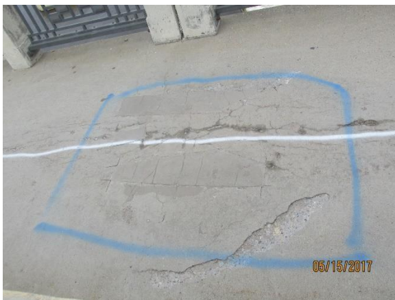
Figure 4.25. Large sidewalk delamination.
