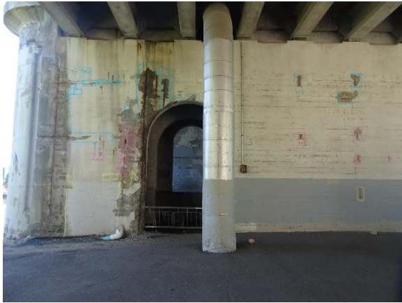
Figure 4.65. Deteriorated concrete on the north face of Pier 8 (outlined in spray chalk).
