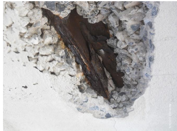
Figure 4.57. Arch rib exposed Melan truss angle at location of poor concrete consolidation.
