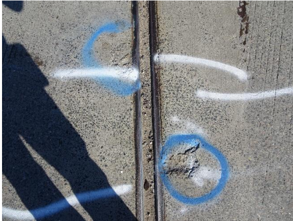
Figure 4.29. Strip seal gland filled with debris. Cracks and spalls are present in the nosing material.
