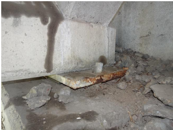
Figure 4.92. North abutment fixed bearing surface rust.
