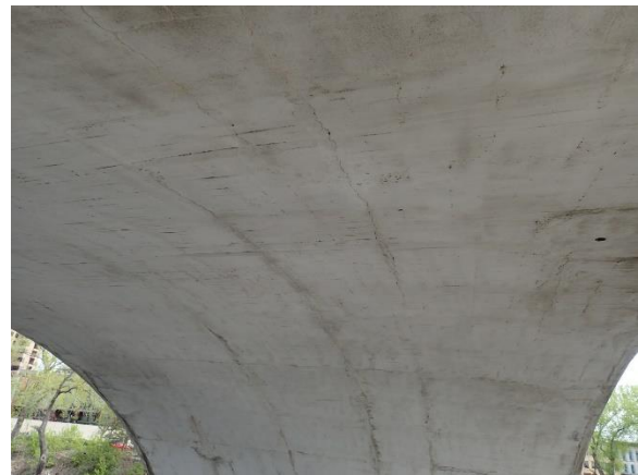
Figure 4.59. Barrel arch underside cracks aligned with Melan truss angles.
