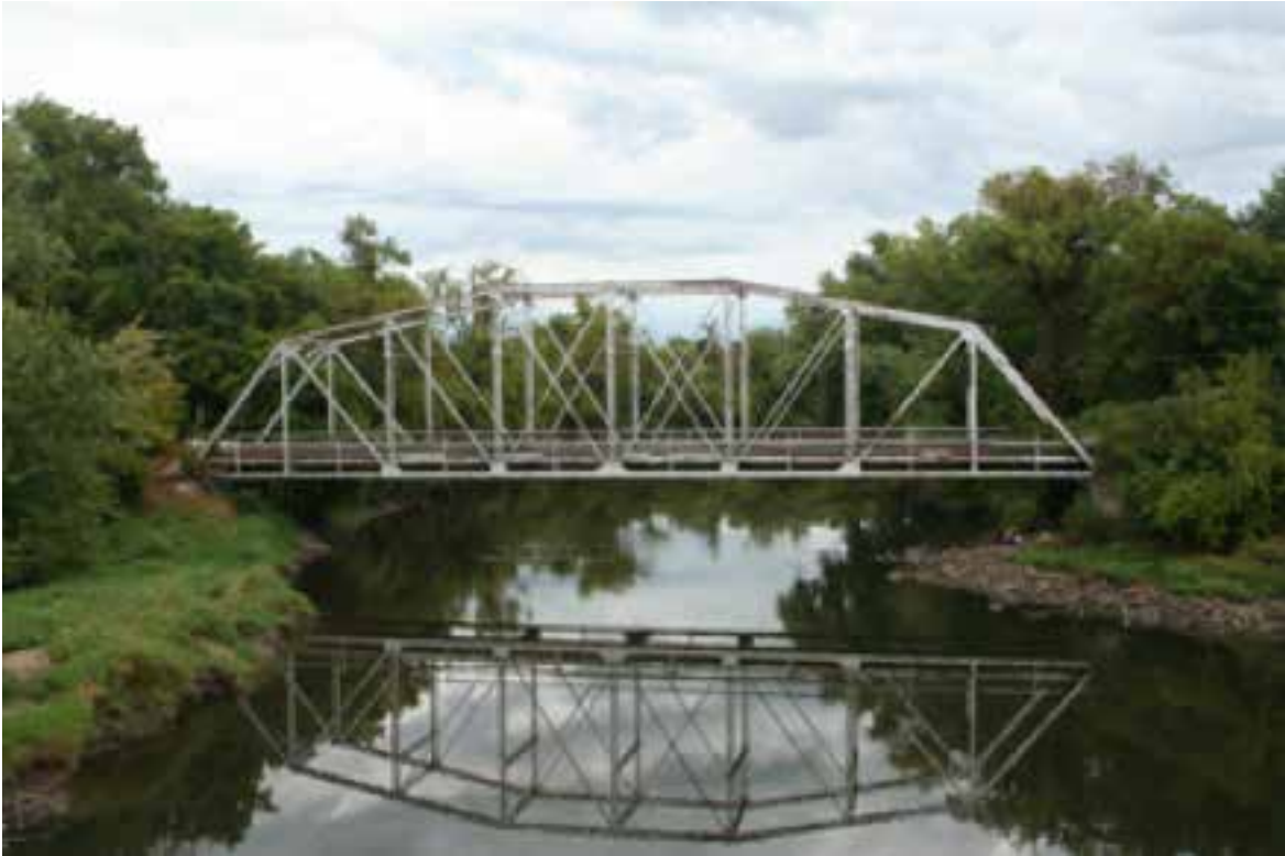
Truss bridge in Waterford Township (Dakota County, MN) Photo credit: Minnesota Department of Transportation
