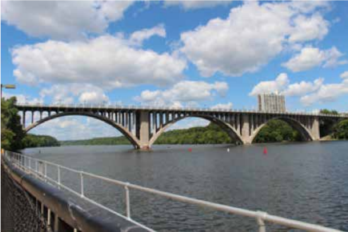
Concrete arch bridge in St. Paul, Minn. Photo credit: Minnesota Department of Transportation
