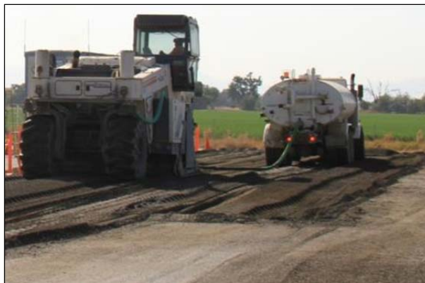
Figure 3.33: FDR-PC: Inconsistent mix on high cement content cells.
