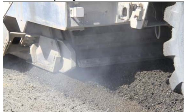
Figure 3.7: FDR-NS: Smoke during pulverization.
